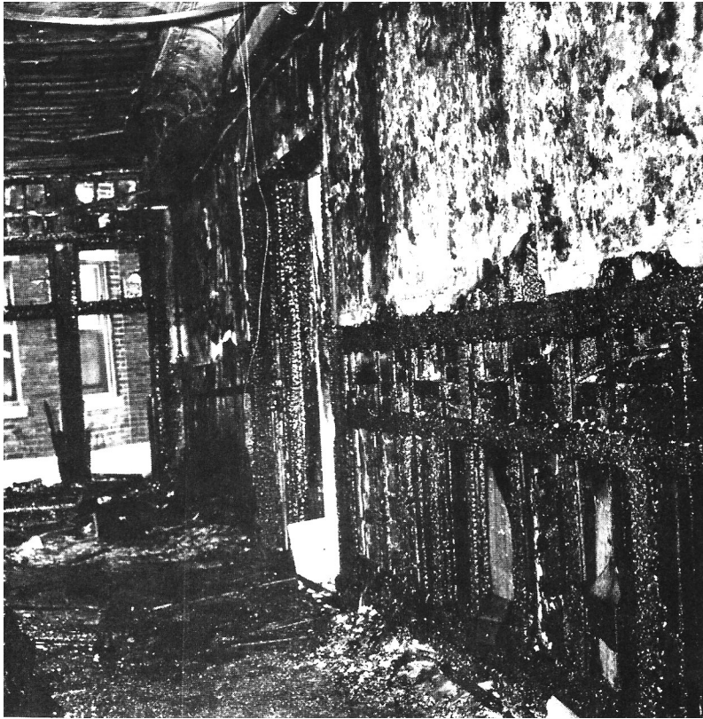
Fire point of origin on the first floor hallway. Photo Courtesy of the NFPA
