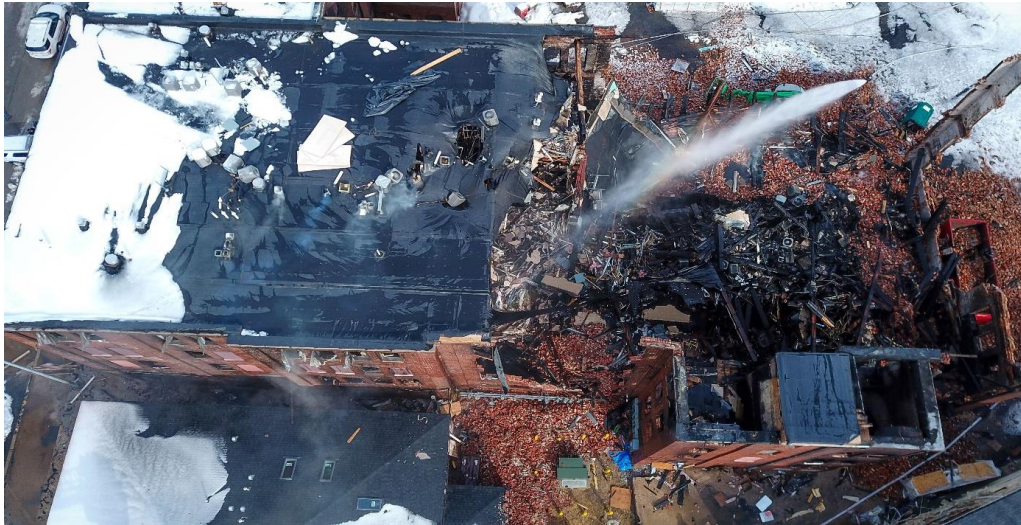
Over view of the collapse areas of the factory. Photo courtesy of The York Dispatch.
